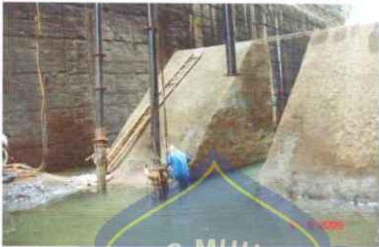
Gambar 7 Euffle Block at Salauli Dam
