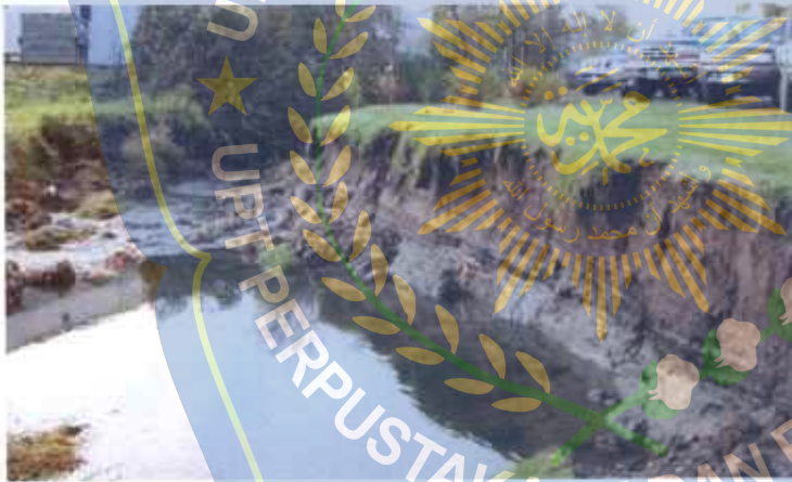
Gambar 1. Erosi tebing sungai
