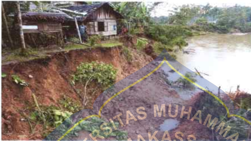
Gambar 8. Erosi tebing sungai
