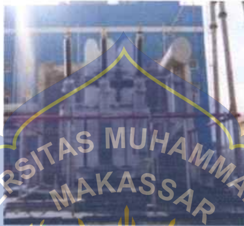
Gambar 4.2 Transformator daya UUP PLTU BARRU
