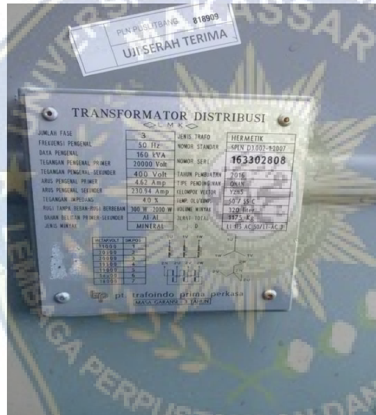
Gambar 4.3 Nameplate transformator distribusi trafindo
