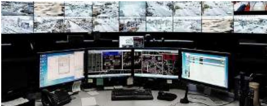
Gambar 9 Ruangan Command Center PTPN IV
