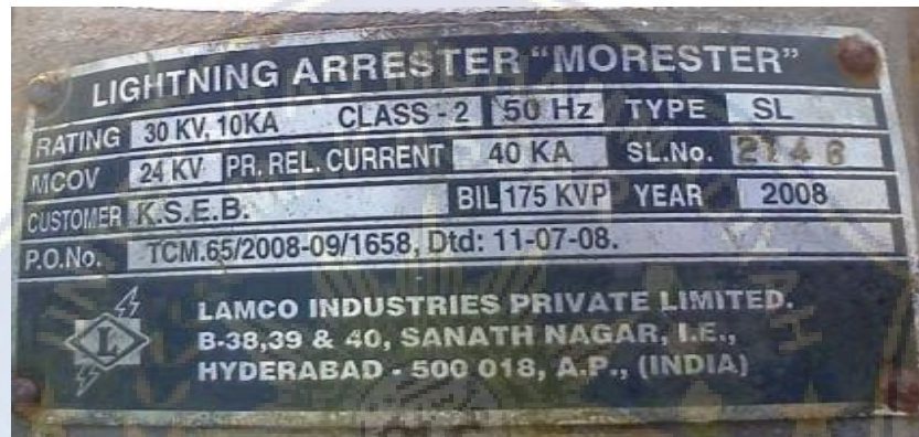
Nameplate Lightning Arrester
