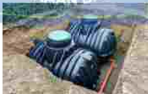
Gambar 3.33 Sistem Ground tank
