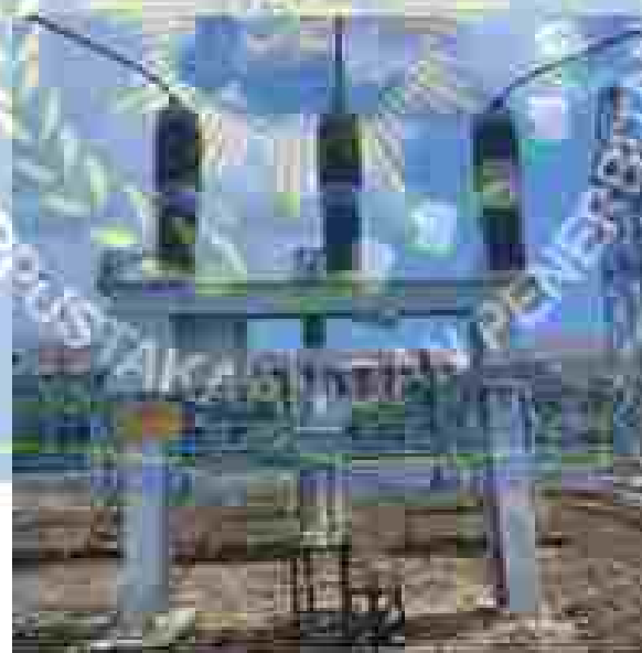
Gambar-2.2 SF6 (Circuit Breaker) sumber: Gi Tallo Lama
