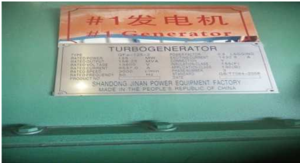
Data Name Plate Generator PLTU Jeneponto (Type Generator)
