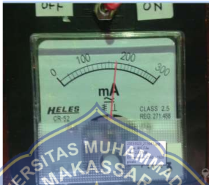
Gambar L. 25. Arus netral lampu TL 30 Watt
