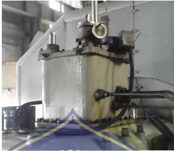
Gambar 16. Governor BTG 1 Power Plant PT. Semen Tonasa
