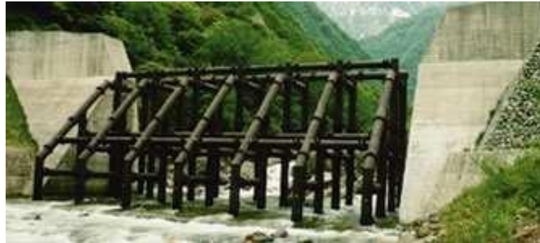
Gambar 8. Cek dam tipe grid pada sungai ikazawa propinsi Niigata Japan (Source: Sustainability Report-Kobe Steel Group Sites, 2011)
